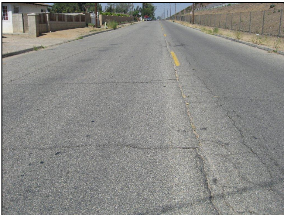
Figure 2D. PCI=56 (At Risk Condition)
