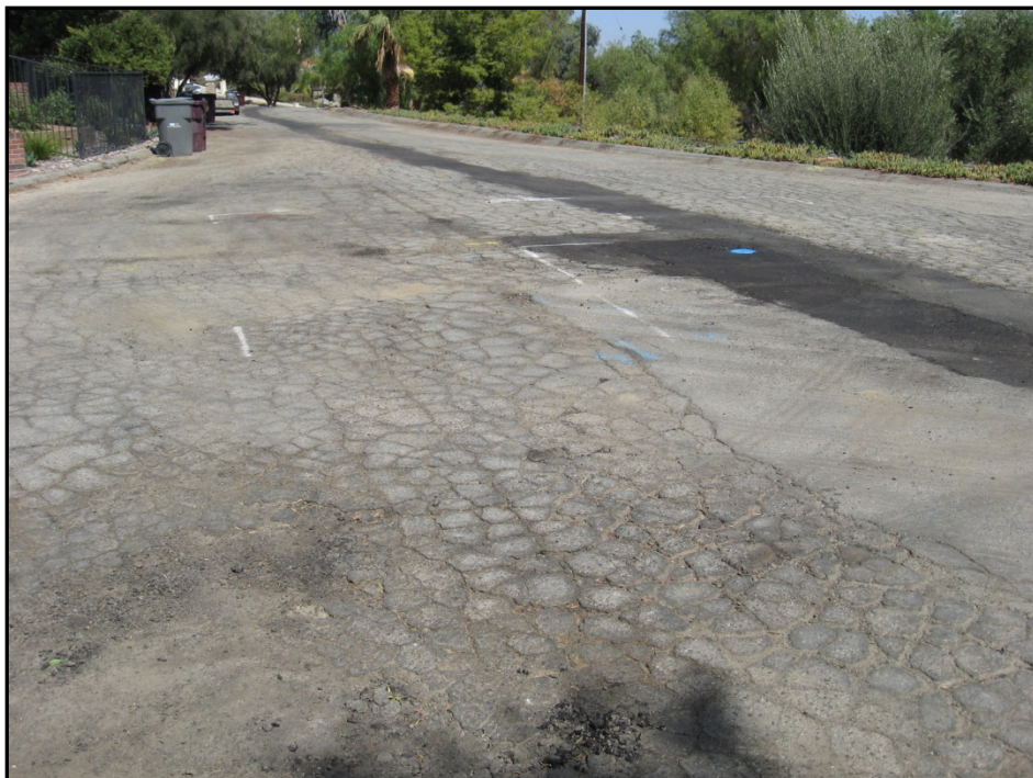
Figure 2F. PCI<10 (Very Poor Condition)
