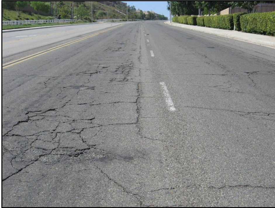
Figure 2E. PCI=30 (Poor Condition)
