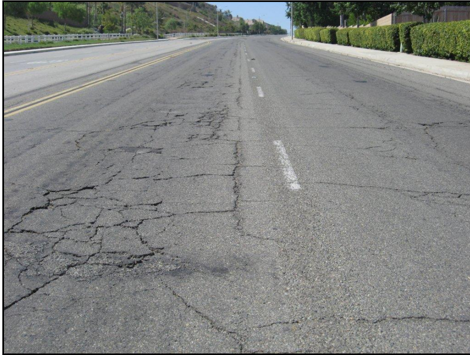
Figure 11E. PCI=30 (Poor Condition)
