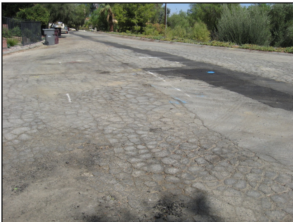
Figure 11F. PCI<10 (Very Poor Condition)
